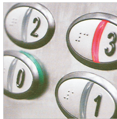
Car Operation Panel
